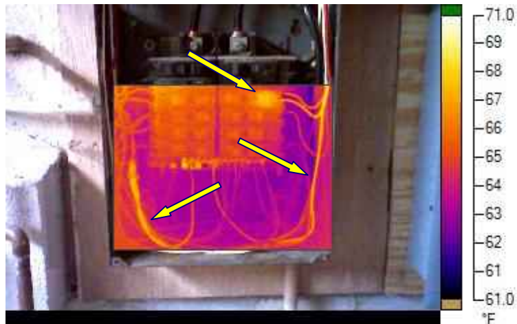
Infrared camera shows one breaker and two electrical wires hotter than the other breakers and wires.
