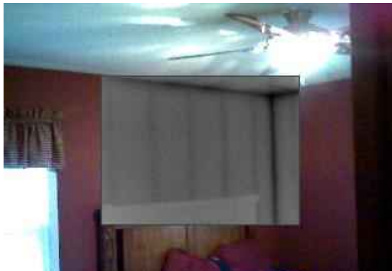
Infrared camera shows the temperature differential on the drywall from the insulation and wall studs.
